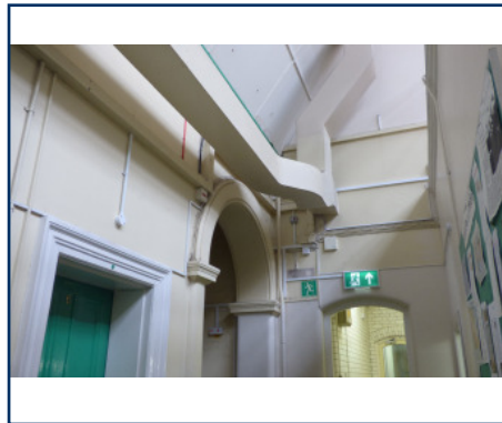
Fig. 33 More service intrusions.
