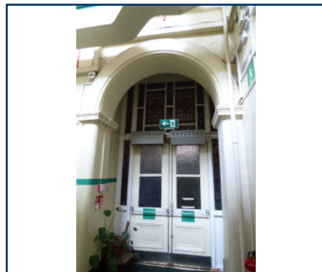
Fig. 34 Original doorway virtually obliterated by services.
