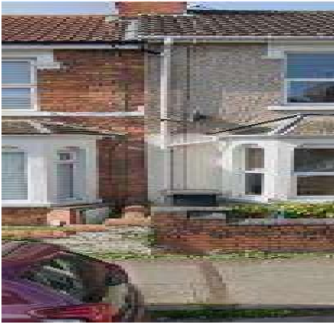
Figure 20 Shared roof drainage downpipe discharging onto the highway footpath in Montagu Street
